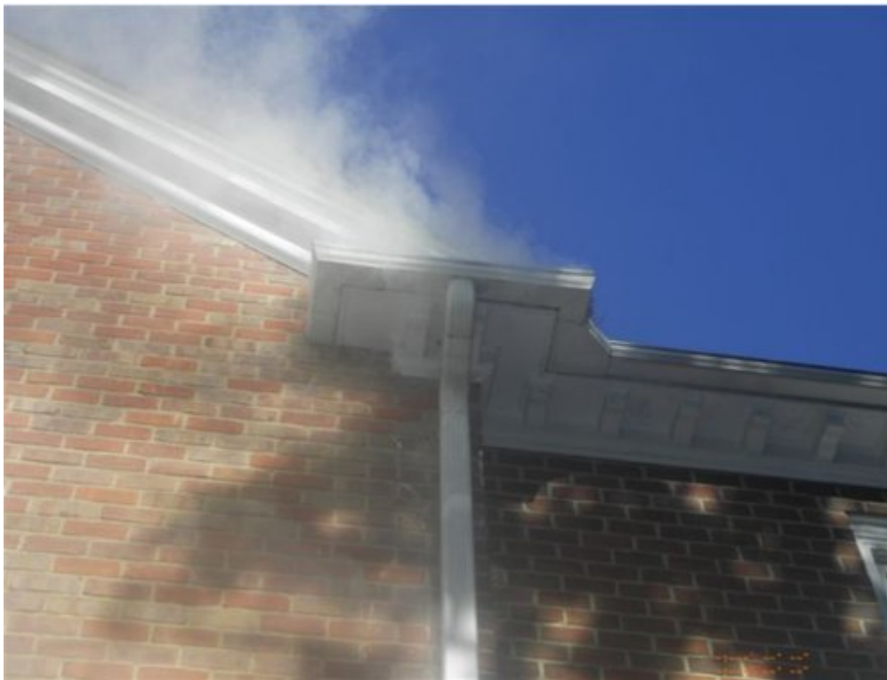
Smoke coming from Roof Leader
