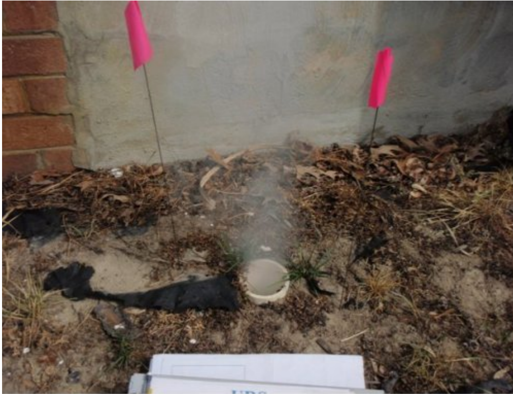
Smoke coming out of Cleanout missing a cap
