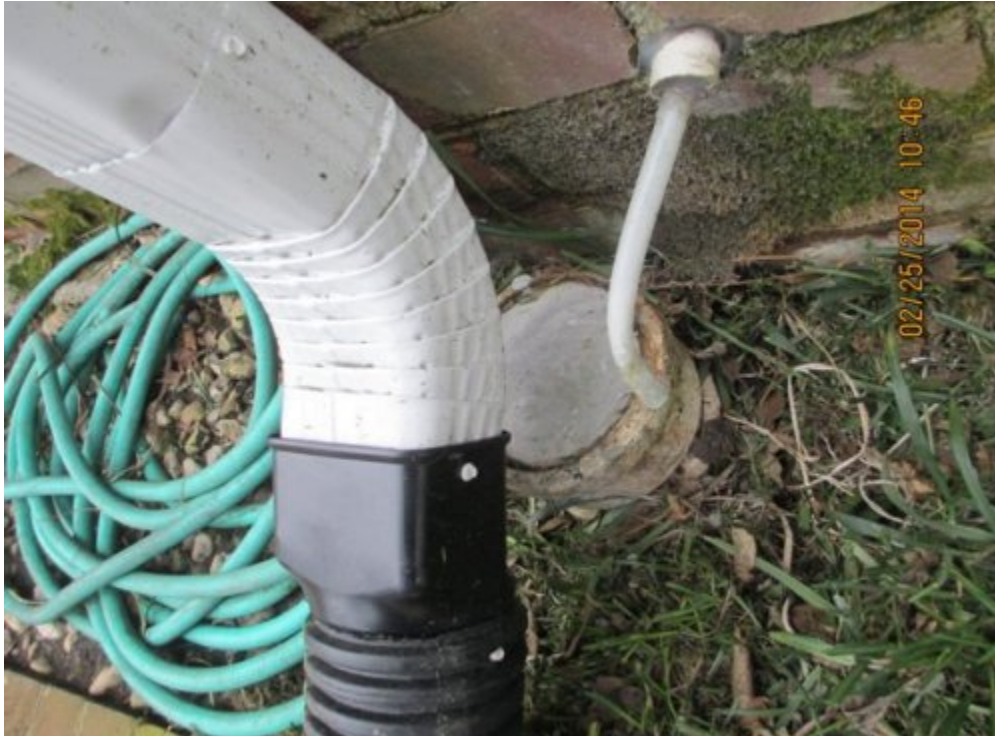
Roof Leader disconnect from sewer system; Former connection to sewer system plugged
