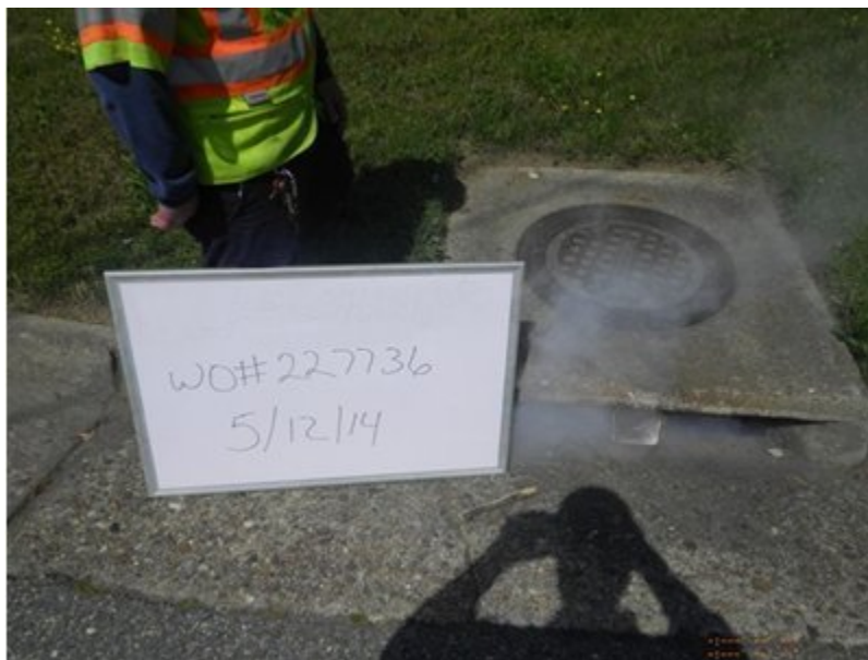
Smoke coming from storm drain cross connection
